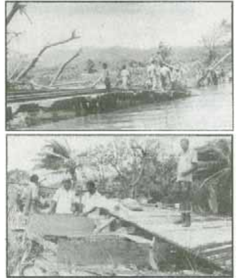
Above: Building collapse - Why?
